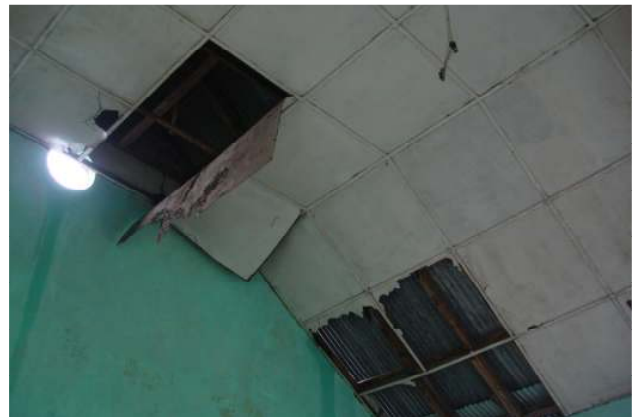
Repairs are needed
